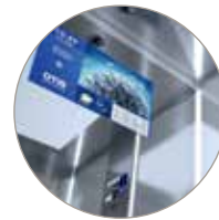
LED lighting: Car Operating Panel
