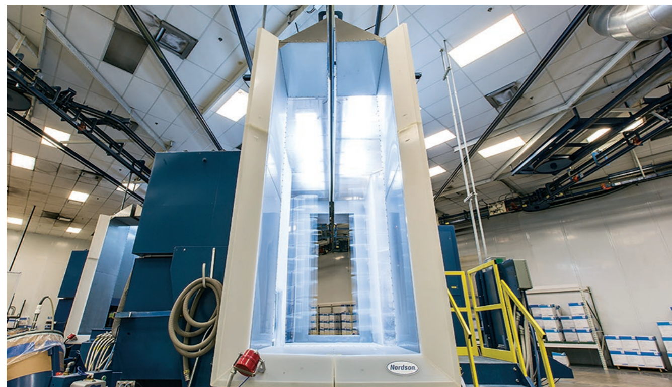
Powder coating line at Middleton, TN plant
